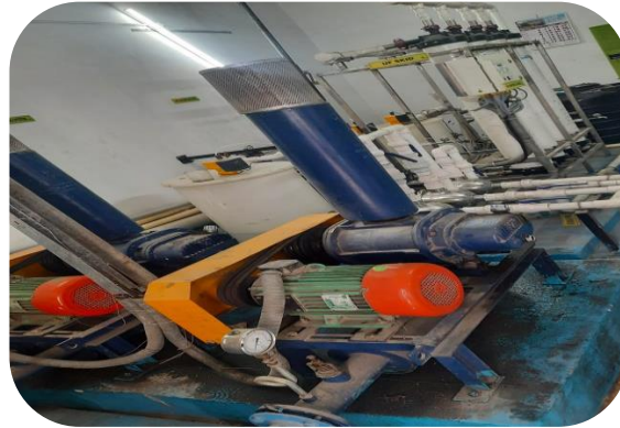
Sewage treatment plant Sewage is pretreated before its let to environment Treated water used for gardening
